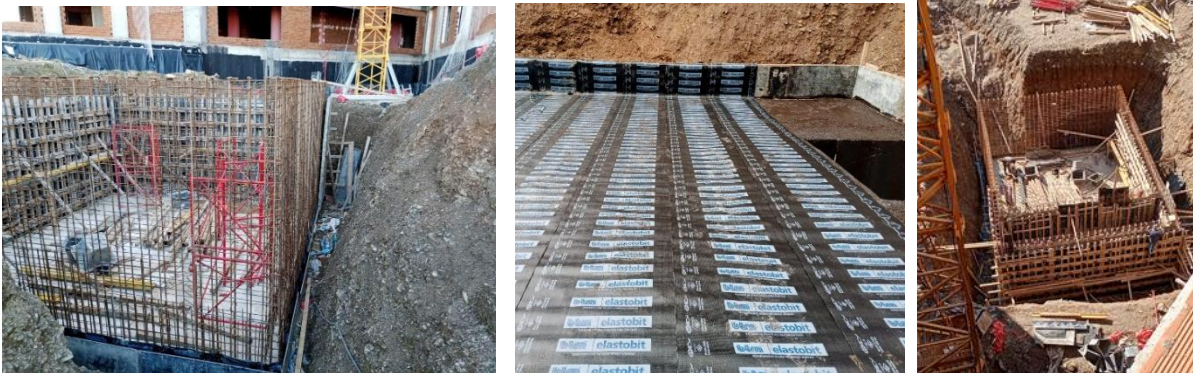
Construction of the 300-tons underground rainwater storage tank at the 15 July Health Campus
