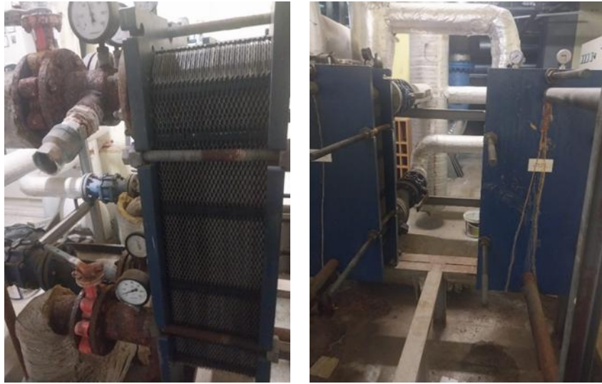
Geothermal Exchangers in 15 Temmuz Health and Art Campus
