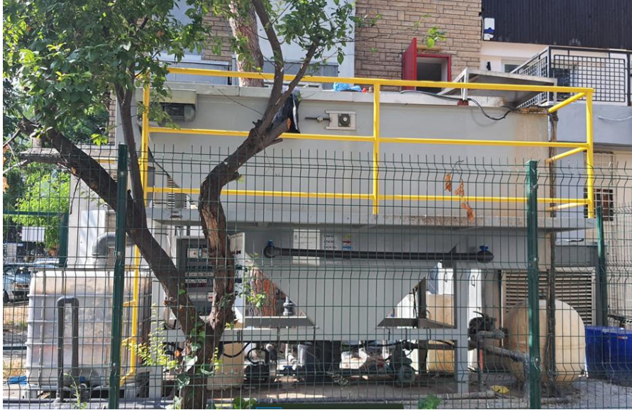
Closed grit chamber systems for pre-treatment of wastewater to be discharged to the sewer system (15 Temmuz Health and Art Campus)
