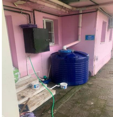
Rainwater harvesting in Bergama Campus
