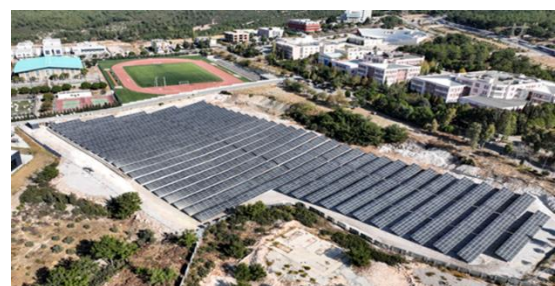
Solar energy panels from Tinaztepe Campus
