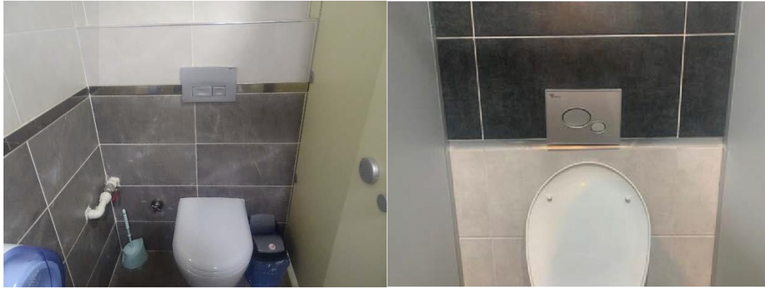
Use of double-stage reservoir systems in various DEU Campuses
