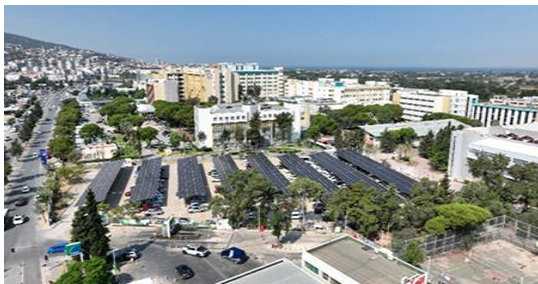
Solar energy panels from DEU Research Hospital
