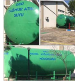
Rain water harvest system
