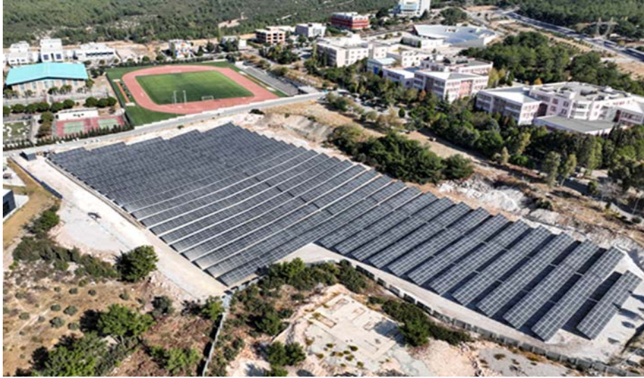
Solar energy pannels in Tinaztepe Campus of DEU
