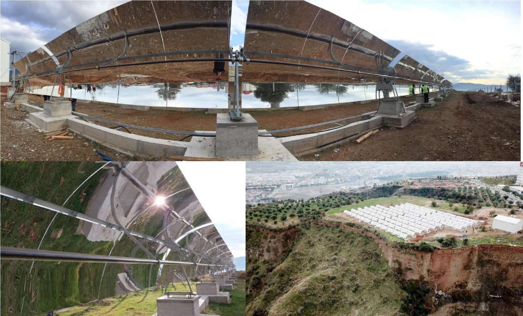
20 modules of the solar collector system PTMx-36 (SOL): Phase 1 Ground installation over separate foundations for each plate
